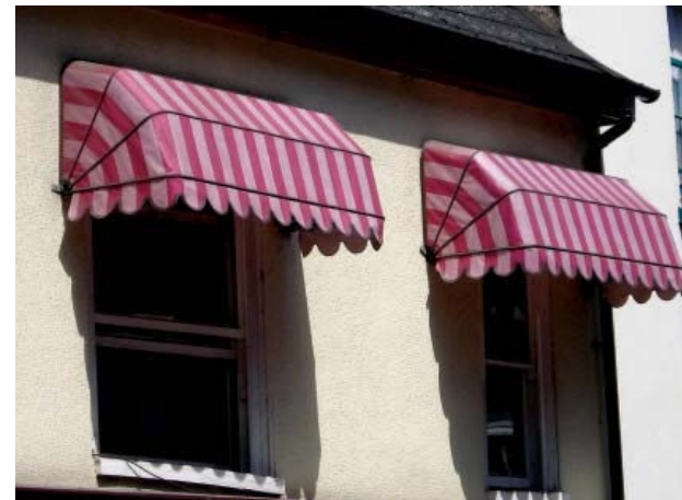
Dutch blinds are generally not acceptable
