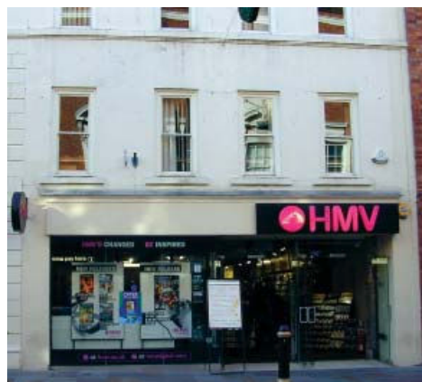
Lettering is garish and its position on fascia does not relate to shop front or building above
